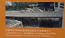
兩條園藝美化高架行人道連接啟德和將軍澳 Construction of elevated pedestrian walkway connecting the Kai Tak and San Po Kong
