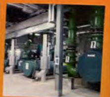
啟德區域供冷系統北廠 Kai Tak District Cooling System North Plant
