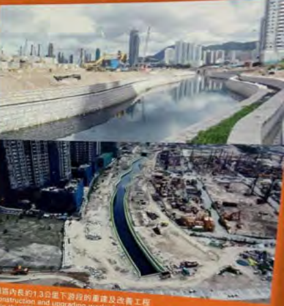
啟德區內長約1.3公里下游段的渠建及改善工程 Reconstruction and upgrading works for the 1.3 km downstream section within the KTD
