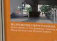
兩條全新行人隧道連接啟德和九龍城及啟德和彩虹 Construction of the pedestrian subway and the Kai Tak and Chui Hung
