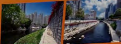
舊大仙洞內一段長約1.1公里啟德河的渠建及改善工程 Reconstruction and improvement works for a section of Kai Tak River measuring about 1.1 km in length located in Wong Tai Sin District
